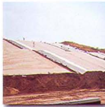
Carbofol® as a base and cap seal in the Soeldershoek Landfill, Netherland.
