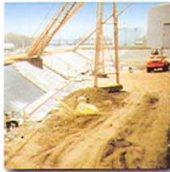
Secondary containment and groundwater protection at a tank farm with Carbofol® geomembranes, Germany.
